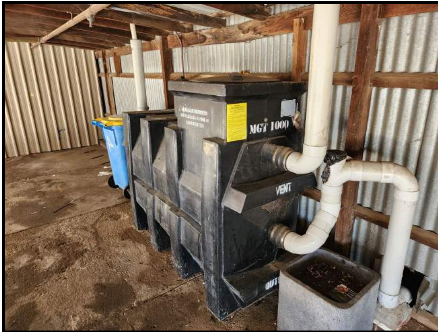
Plate 7: Photograph of grease arrestor in garage/carport area beside Ray Ray's Diner.
